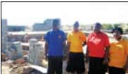
Thesate Church in Pitsoane was destroyed by wind last March. Now the church is pleading with the community to help them rebuild it. Pastor Rodney Mayimbe of Thesate Church, Administrator, Justice Mathomo, Pastor's wife Constance Mayimbe, and Financeer Enoch Machebe.
